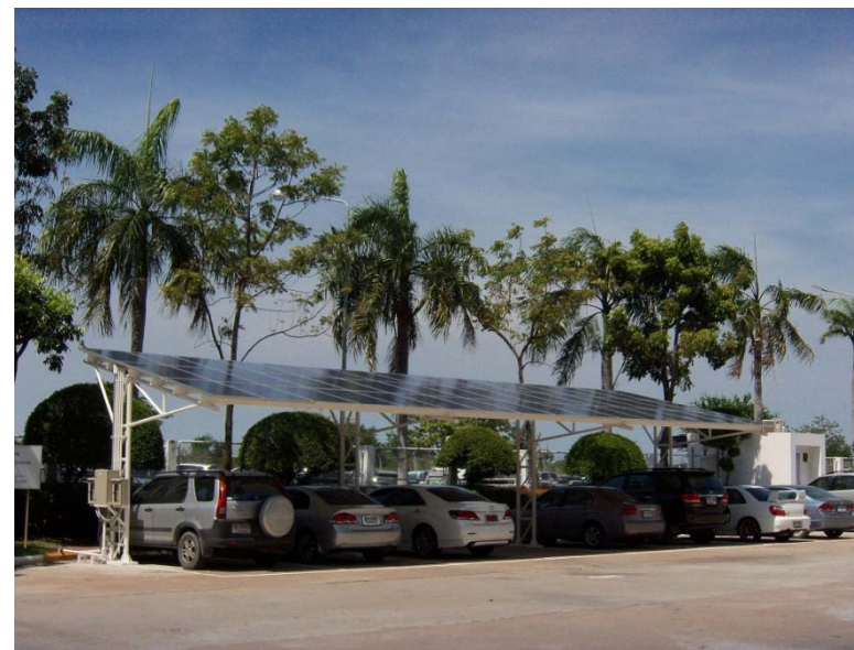
11 kWp, Delta Electronics (Thailand) PCL., Samutprakarn. (2011)
