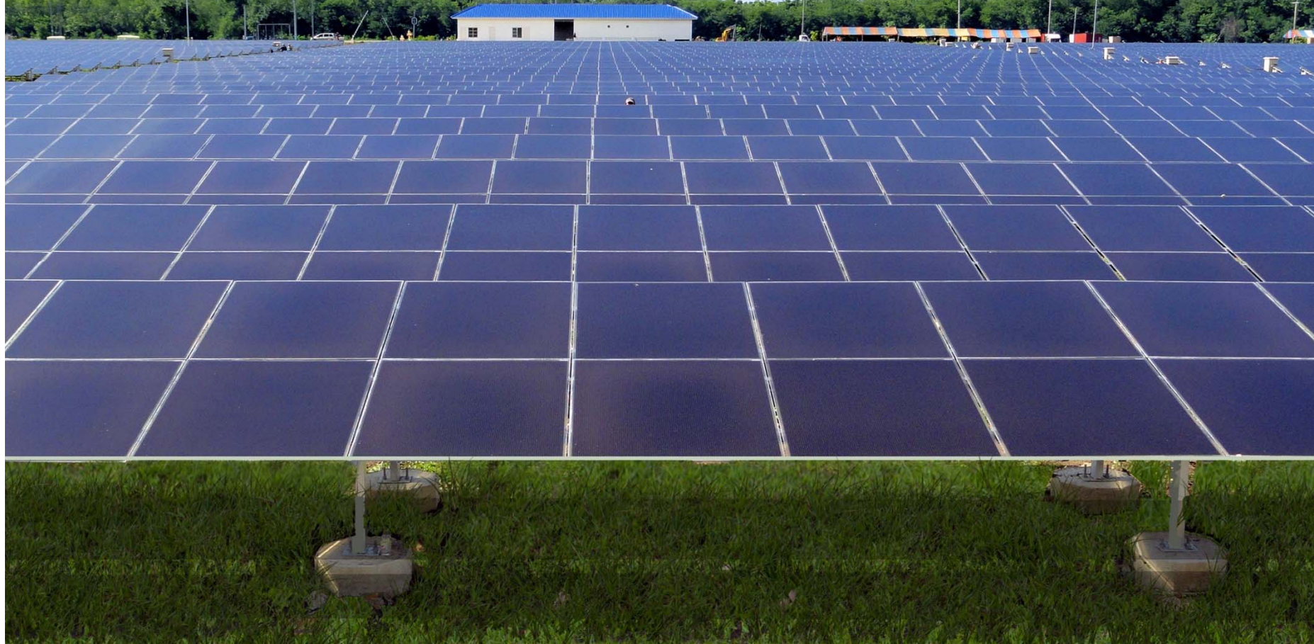
1.65 MWp, Solar Park Co., Ltd., Lopburi (2011)
